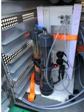
Figure 5.5 – In-situ measurement of the NO 2 adsorption efficiency. Airyx ICAD measurement device installed in a filter column (phase III).
